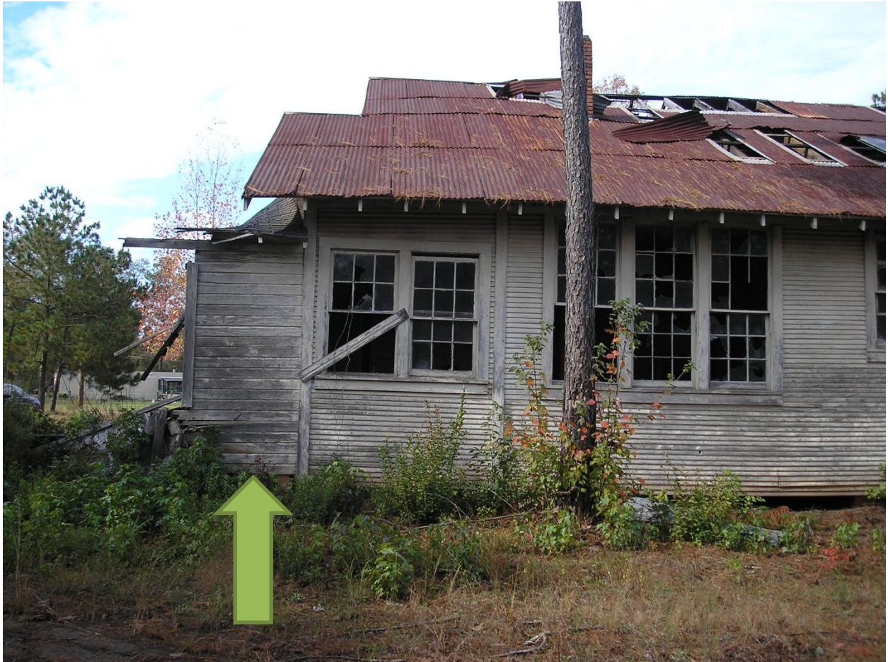
1925 Building, east elevation, south area. Non-Period addition (green arrow) has been removed.
