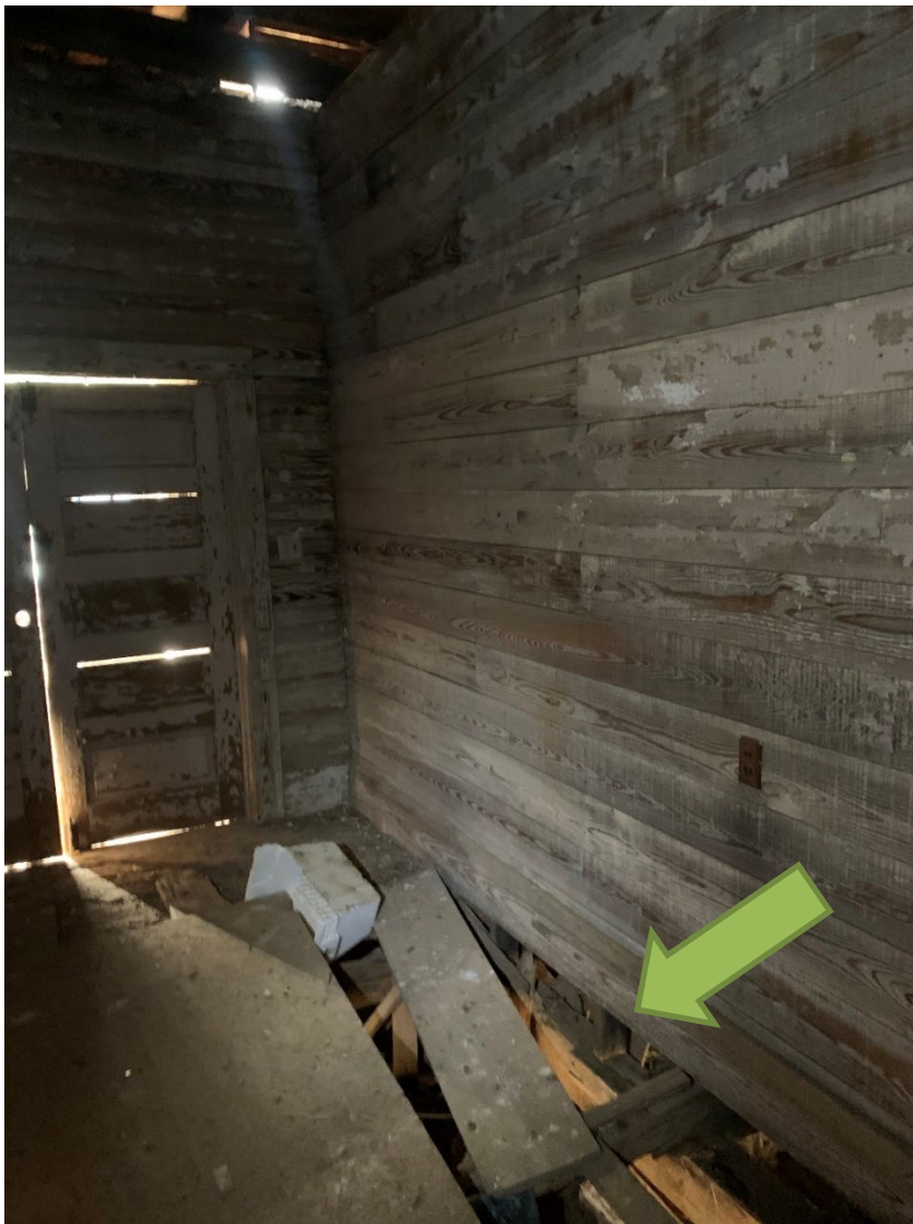
Typical condition of interior studs connecting to sill. Flooring is interrupted.
