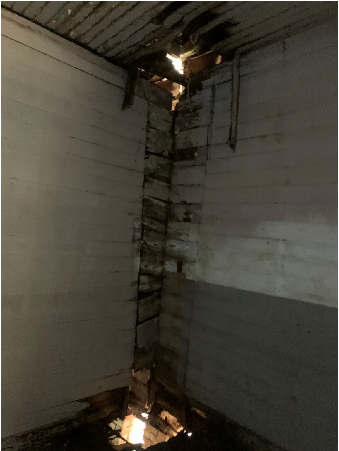
Excessive deterioration at interior wall corner.
