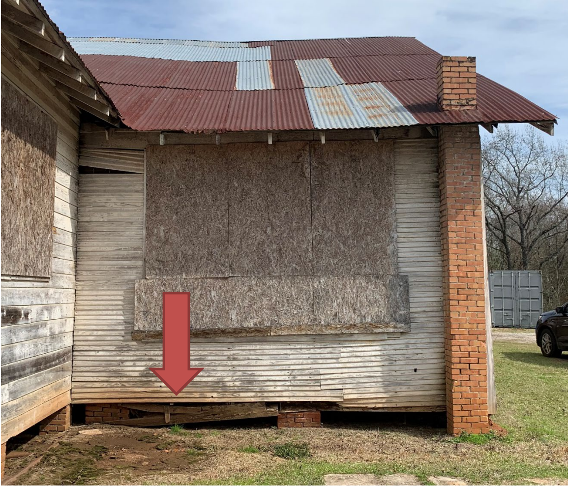
West elevation. Damaged piers and failed sill.
