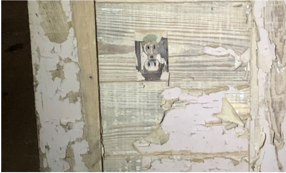
Original ebonite receptacle cover plate.
