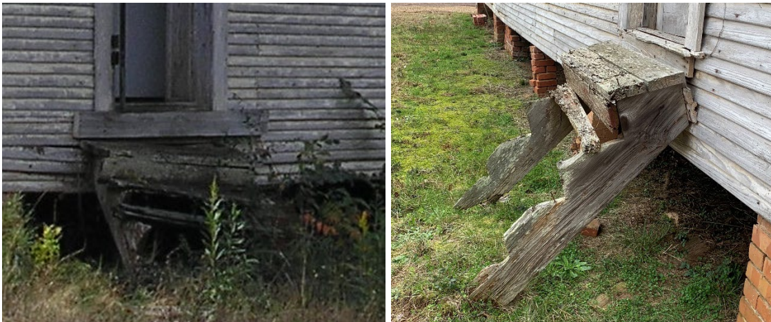
1925 Building. North elevation, remains of exterior stairs. West (2008 photo) and east stair.
