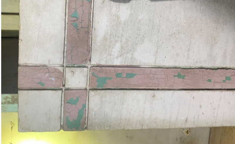
1925 Building. Room 104 – North end of room. Colors indicating millwork was painted twice.
