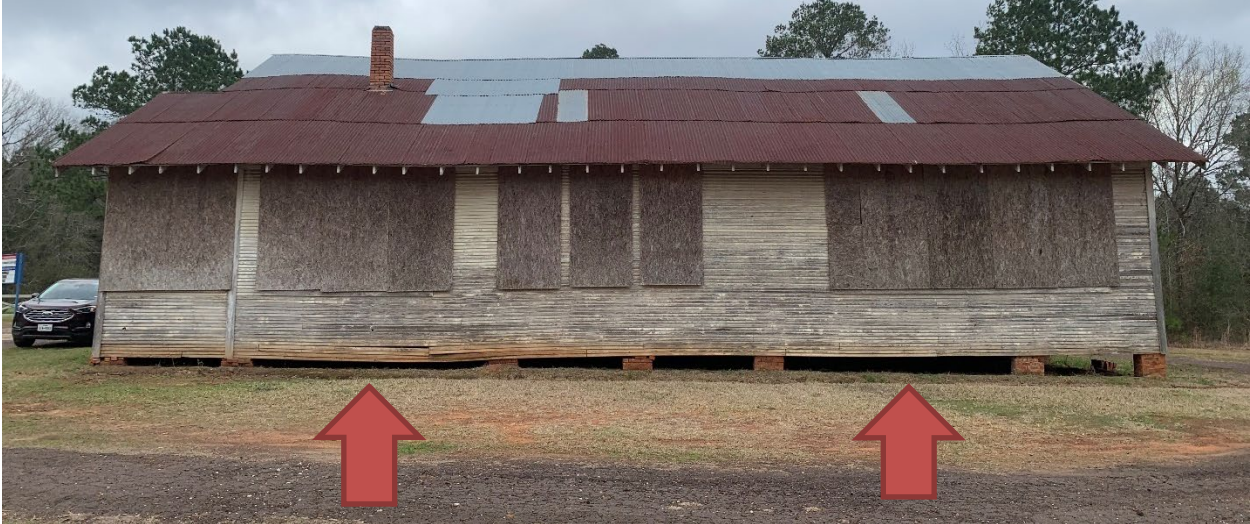
East Elevation. Missing piers.
