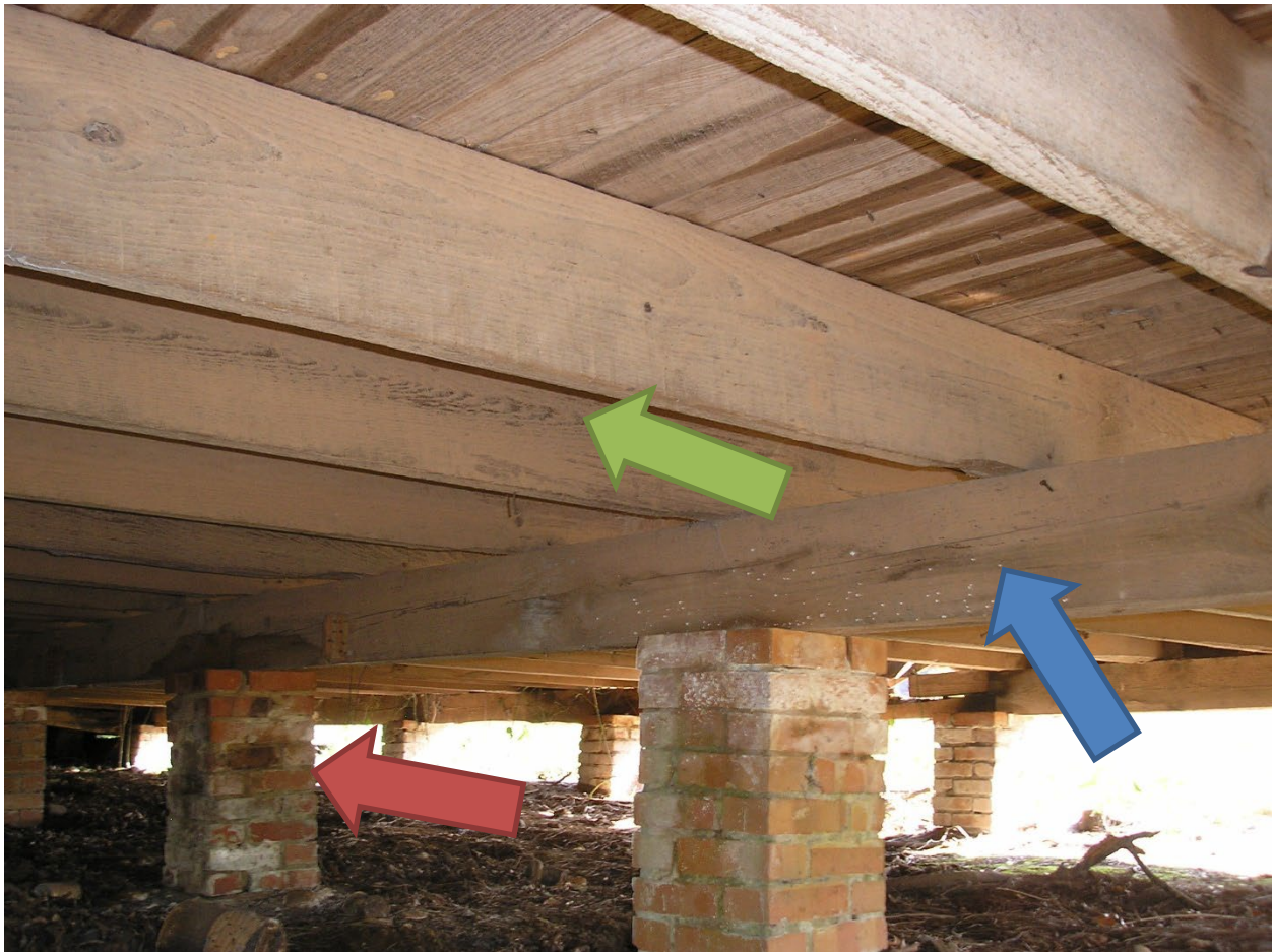
Foundation system. Piers (red arrow), Sills (blue arrow), and Joists (green arrow).
