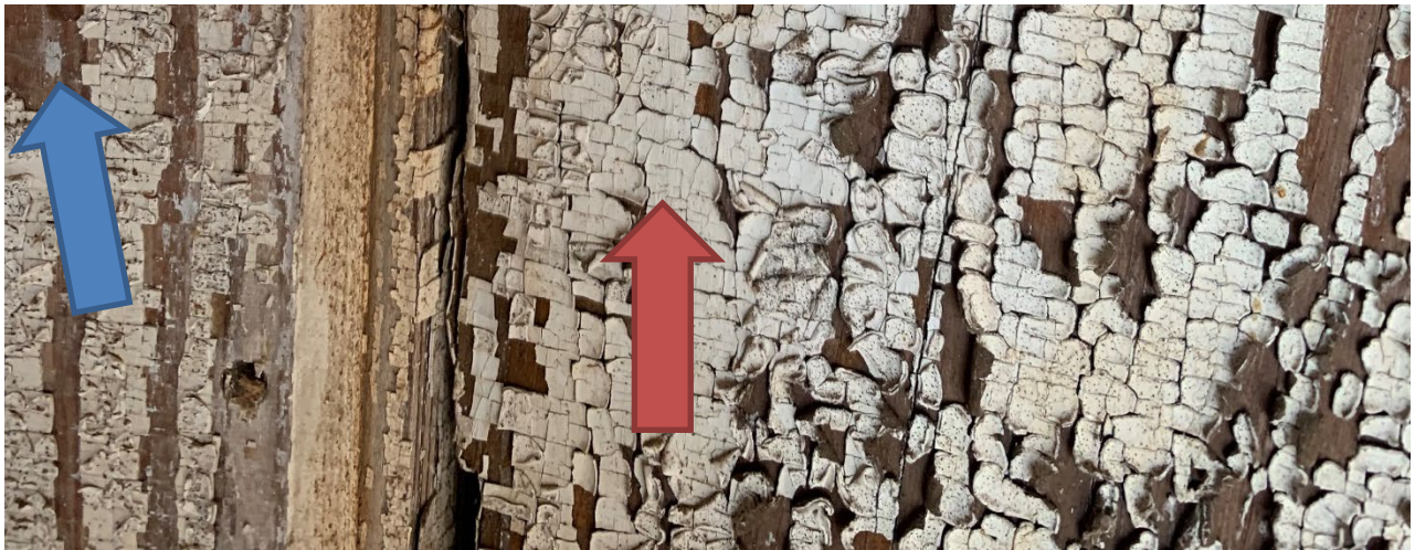
1925 Building. Remains of 1 st generation white (blue arrow), 2 nd generation white (red arrow).
